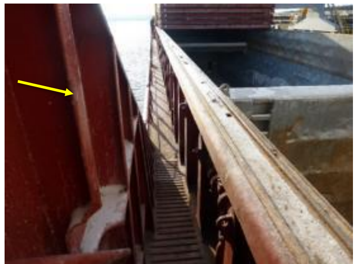
Eductor valves on hatch coaming.
