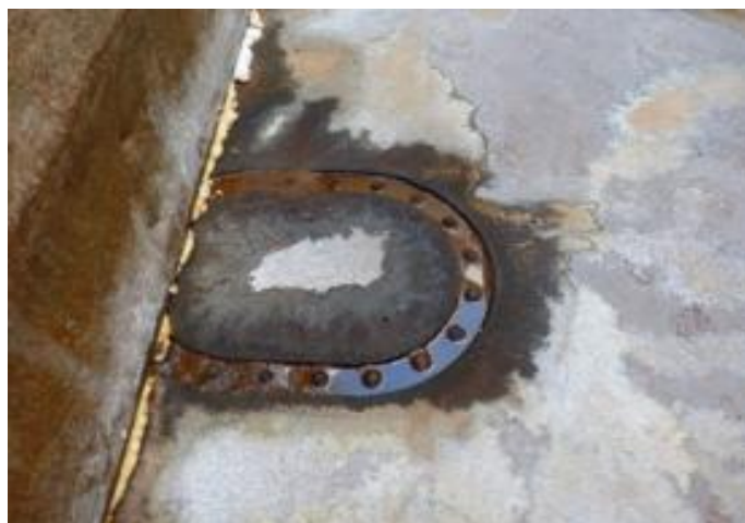
Water on manhole cover.
