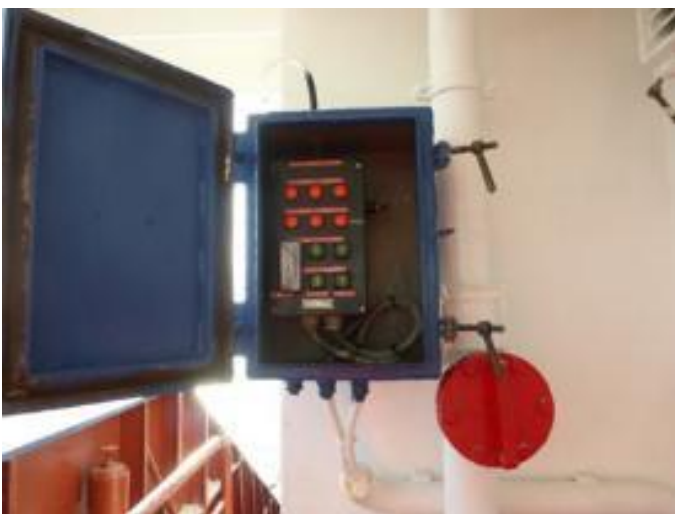
Bilge eductor operating console.
